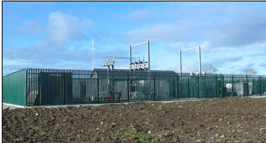
Plate 4-11: Typical Substation Compound
